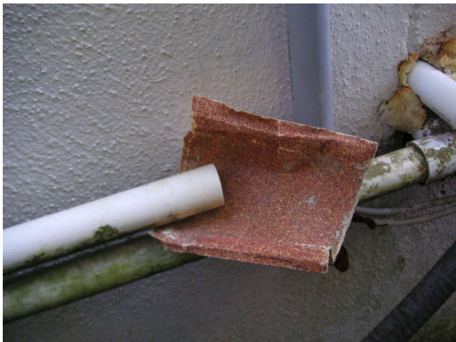
I decided to return the new PVC I bought, so I cleaned this old pipe up rather than replace it.
