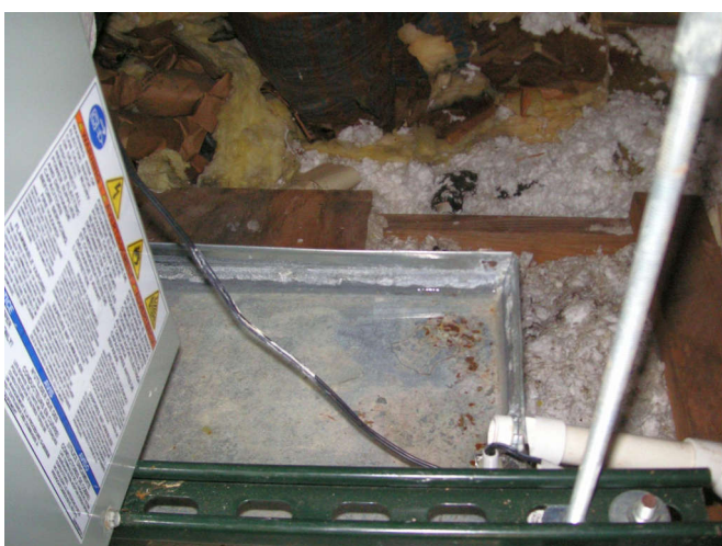
Back in the attic, the overflow pan already has water in it after just one day.
