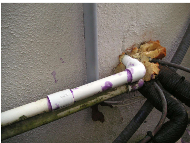
I repair the cut out elbow and make sure the old pipe outlet is where I want.
