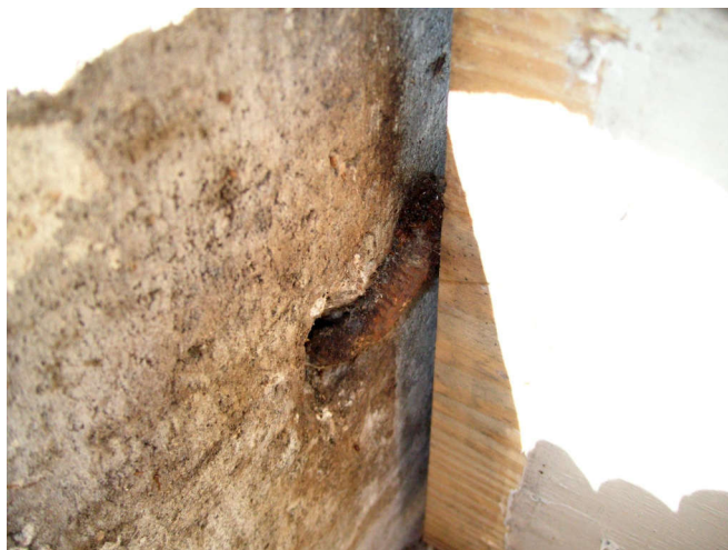
I went to sand the boards on the house, and saw this chunk of rebar bent over and in the way.
