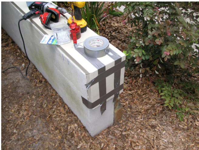
Four strips of duct tape held the end cap while I drilled and screwed in the Tapcon fasteners. What happened to the good duct tape?
