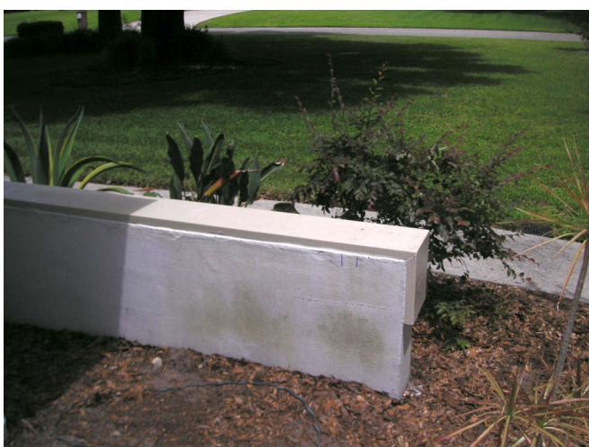
The wall looks good. It will get puttied and another color coat.
