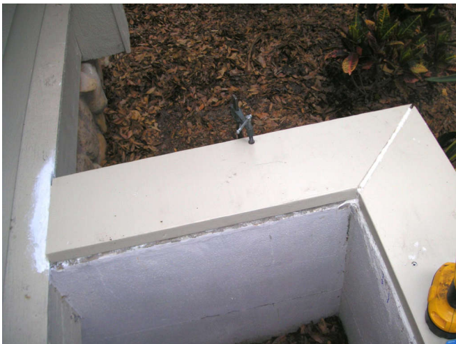
A long clamp held the short top board in place. I had to pull the board up twice so I could mark where the web of the cinder blocks was. That is where I needed to drill for the screws.
