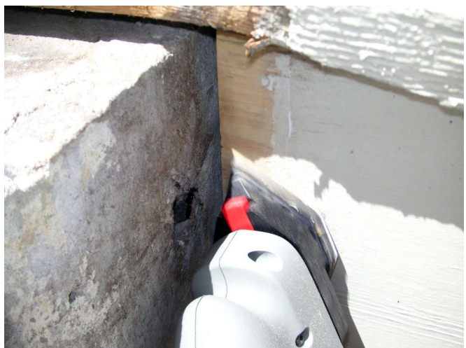
With the rebar gone, I can use the profile sander to clean up the existing boards.
