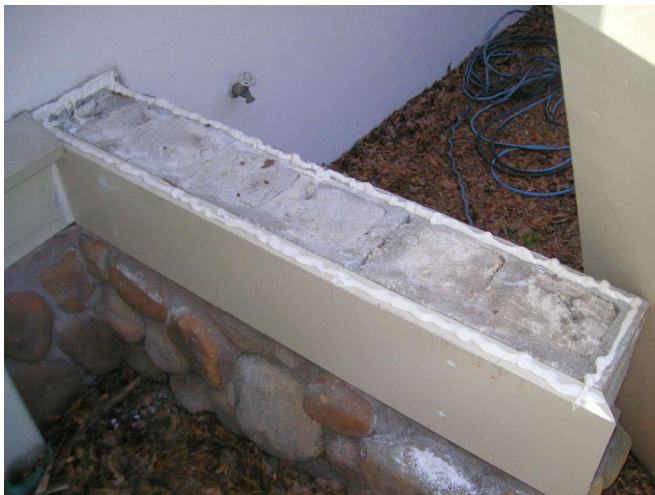
I caulked all around the top to seal the wall from rain and moisture. This got to be a mess.
