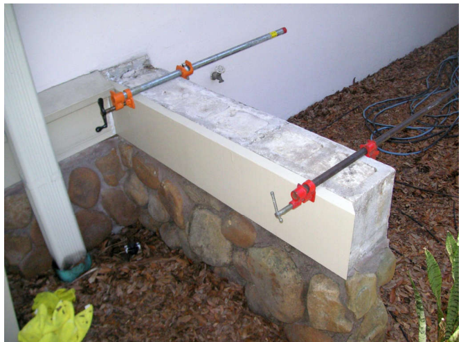
This time I am not going to screw the lumber together. I will just screw the three separate pieces to the cinder-block wall.
