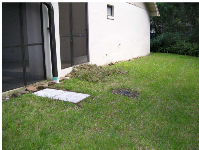
I took up so much dirt with the trenches I could even pile some at the back screen room door.
