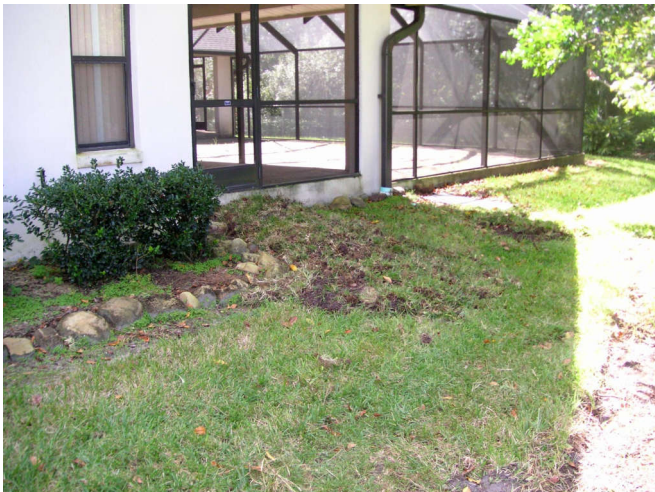
Then I used the dirt and grass to build up the area around my screen room door, as well as a French drain box for the screen room gutter.
